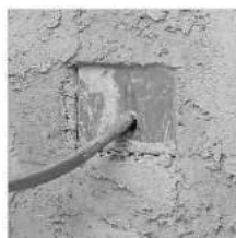
Stucco covering the bracket is chipped away.
